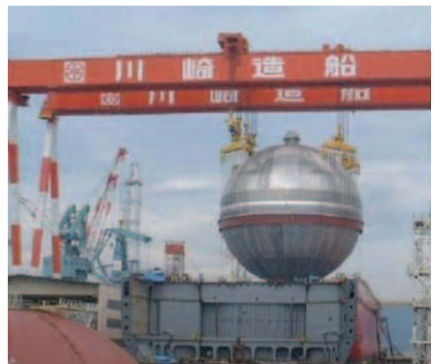
Figure 2: A spherical aluminium LNG container vessel being mounted onto a ship hull using a gantry crane [4].
