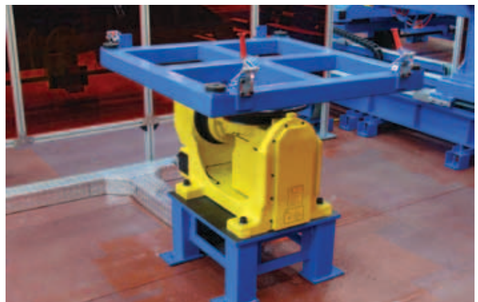
A two-axis manipulator installed in order to improve access to some of the more complex components and to achieve as much flexibility as possible.
