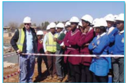
Tiaan Bowman (site engineer at Ninham Shand), explaining construction activities of the Sunderland Ridge Wastewater Treatment Plant near Centurion to the selected students from eight high schools in Atteridgeville in Pretoria.
