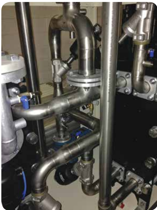
"Duplex stainless steel is becoming more important in the chemical industry because it performs well in high temperature conditions," says Lawrence
