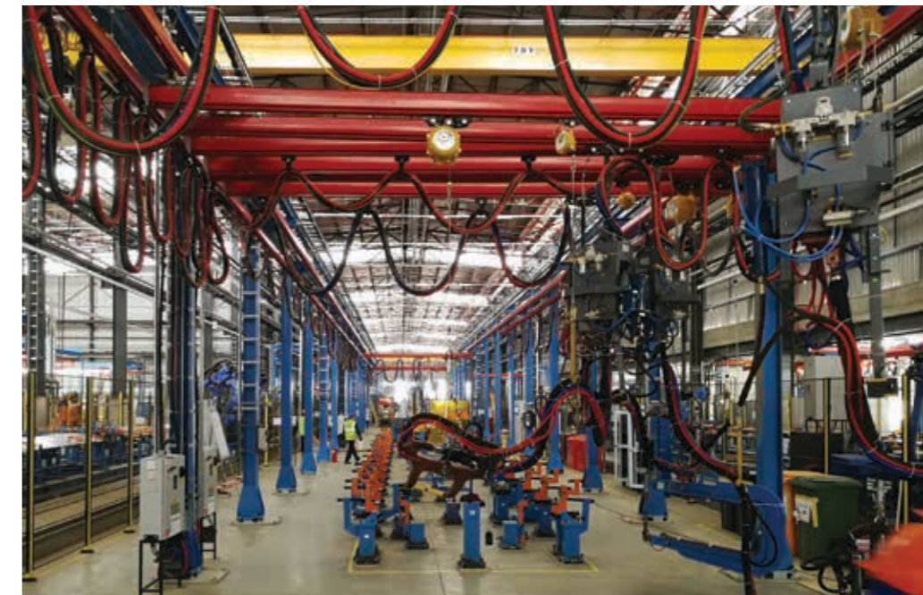
The Underfloor Mainline showing a Nash welding gun balanced on the KBK overhead rail suspension system.
