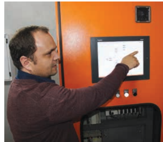
Electrical systems integrator, Brian Cooper at the main control HMI. Pump speeds are controlled via VSDs to prevent overspeed and to convert the electricity produced for compatibility with the city's power grid.
