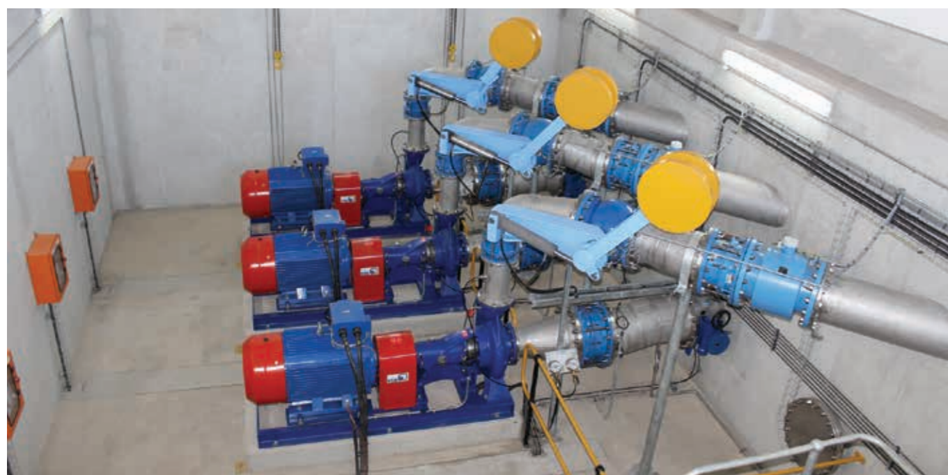
The Drakenstein Municipality's Leliefontein pump and turbine station (PaT), which pumps water to Paarl for one dry month every year, while generating 57 kW of electricity by running the pumps as turbines, for the remaining 11 months.
