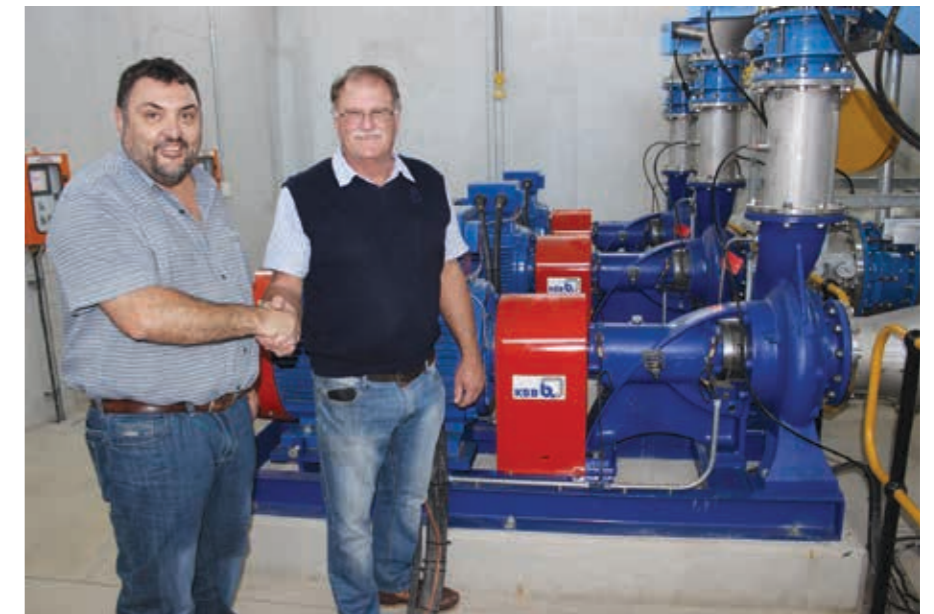
Kiewiet Viljoen, projects director for Hidro-Tech systems and Drakenstein Municipality engineer for water operations, Hein Henning, at the KSB pump and turbine station (PaT).
