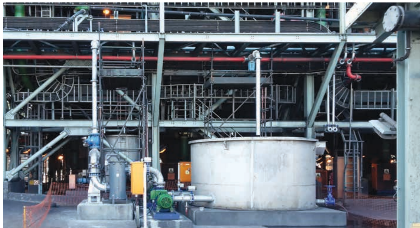
To ensure long-term longevity and availability of the GG7 and GG8 mega-plant at Grootegeluk, Thuthukani Engineering has deployed a turnkey, fully automated and centralised gland service water system.
