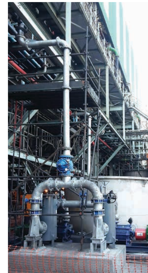
The gland service water pump system for Grootegeluk is a centralised system supporting 44 pumps, from a single tank with two supply pumps, one operational and one on standby.
