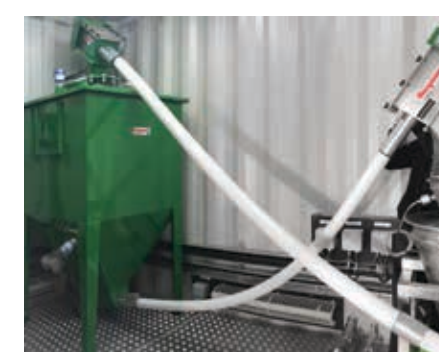
The 5.0 m long flexible screw conveyor from the bulk bag discharger moves the carbon powder to the surge hopper (left), from which the second 3.5 m long flexible screw conveyor moves the powder to the intake of the Transvac ejector (right).
