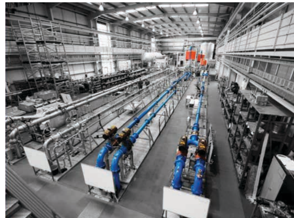
The National Engineering Laboratory's (NEL) flow test facility in Glasgow, UK.
