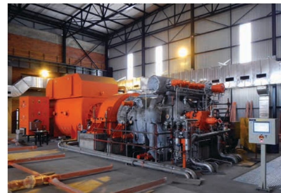
A 48 MW multi-extraction condensing steam turbo generator set, with associated auxiliary systems, used for cogeneration in the pulp and paper market.
