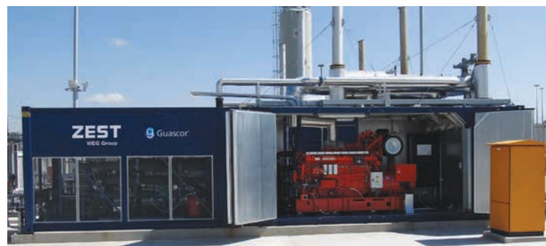
A containerised gas generator set with controls and a heat recovery system for producing energy from treated biogas in the wastewater treatment industry.
