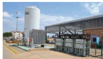
Air Products unveiled its state-of-the-art Dissolved Acetylene facility in Midvaal in October 2018.
