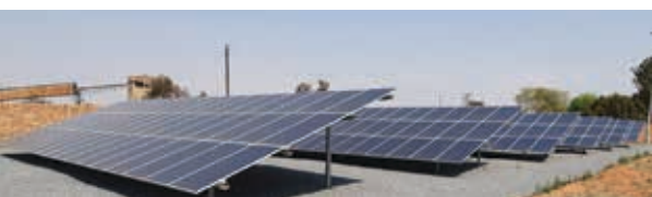
Air Products' Midvaal Dissolved Acetylene facility has a ground-mounted, automated solar system consisting of 306 panels that can generate approximately 170 000 kWh per year.
