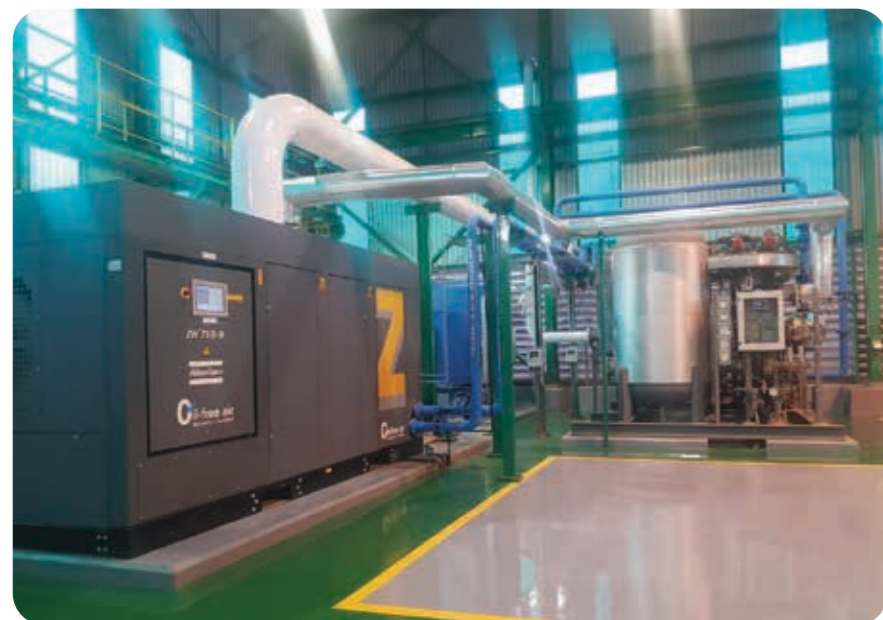
Most recently, Lesedi has now completed a compressed air plant expansion project in Mozambique for the South32 Mozal Aluminium Smelter plant.
