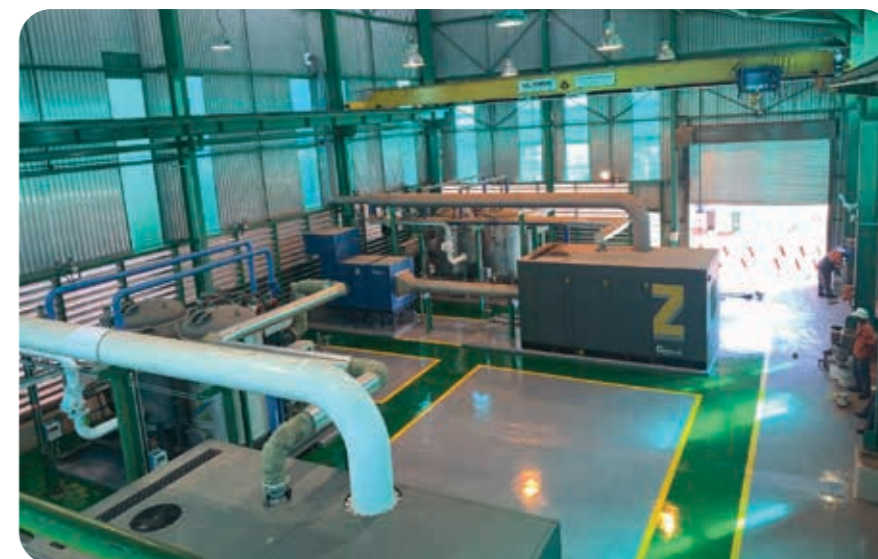
For the Mozal AP3XLE compressed air expansion project, Lesedi was tasked with upgrading the compressed air installation plant through the addition of an additional compressor with its own heat of compression dryer.
