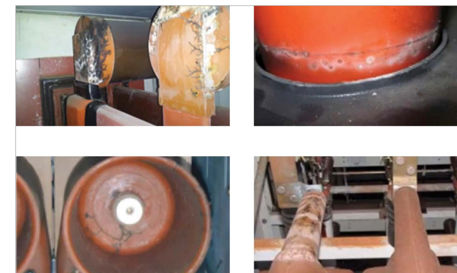
Partial discharge (PD) plays a key role in insulation failure. The physical signs that PD is occurring include, amongst others: the smell and presence of Ozone (O 3 ), a burnt wire smell; discoloured trails along insulation; and carbon tracks.
