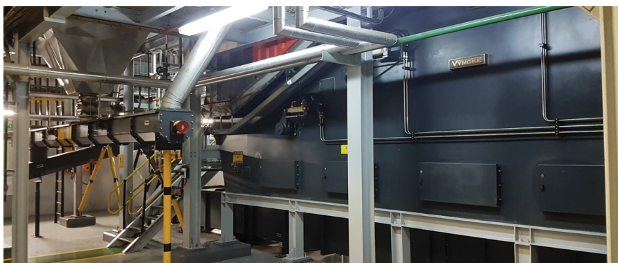
An AES-managed biogas plant.
