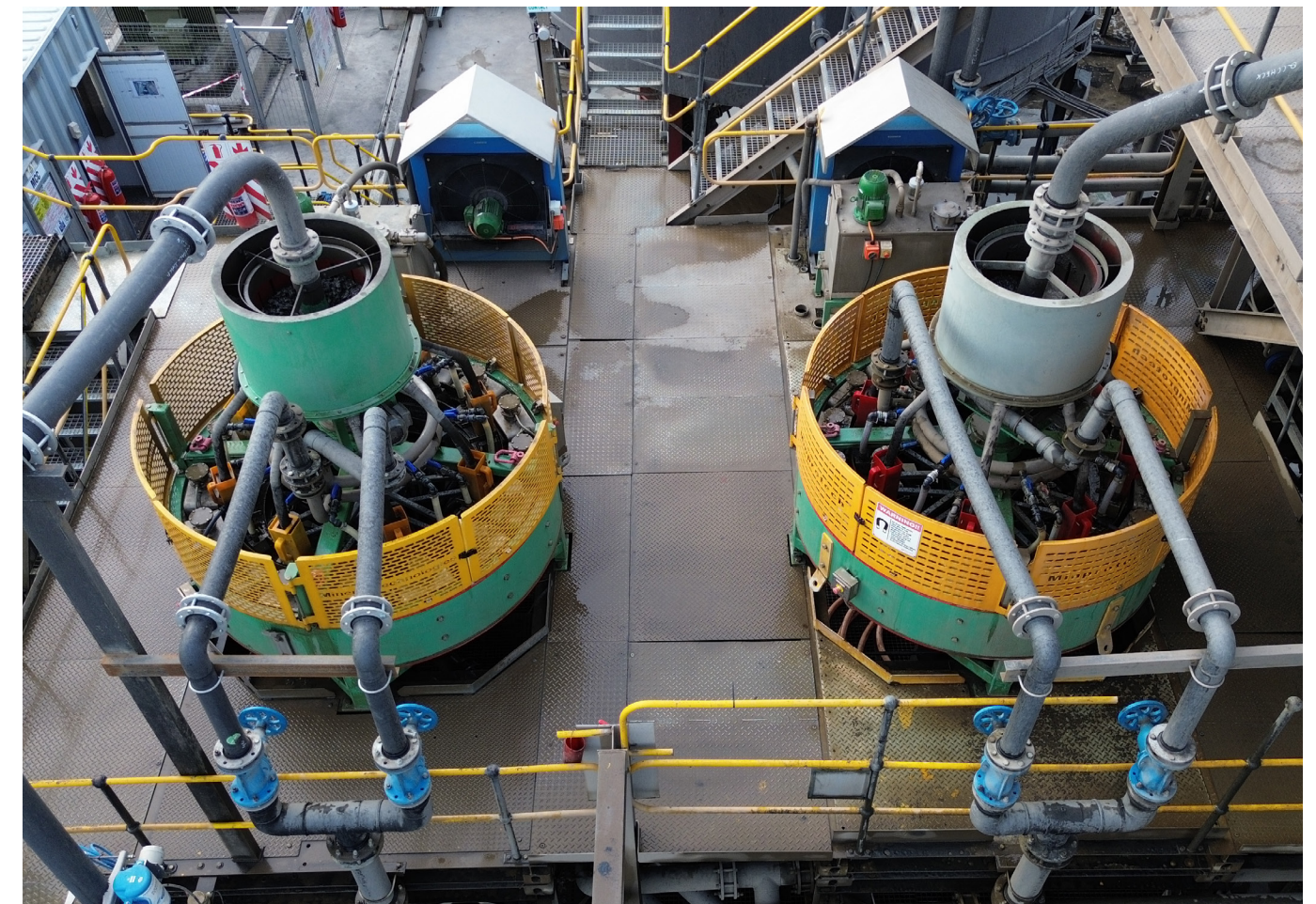
Minprotech specialises in the use of Australian-manufactured WHIMS magnetic separation technology to build and operate successful chromite fines recovery plants.
