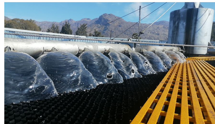
A view of a trickle filter plant delivered to a fruit producer. The first phase of the plant was delivered at the end of 2024 and WEC Water recently commissioned Phase 2 and 3 to enable the total treatment capacity to be increased to 3.9 MLD by 2026.
