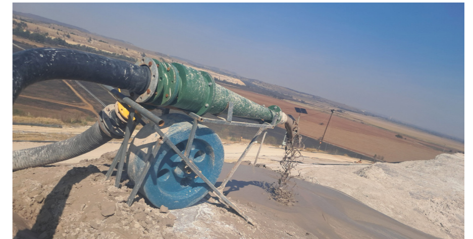
Prioritising the cyclone selection choice allows mines to fine-tune their tailings strategies to achieve both operational and sustainability targets.
