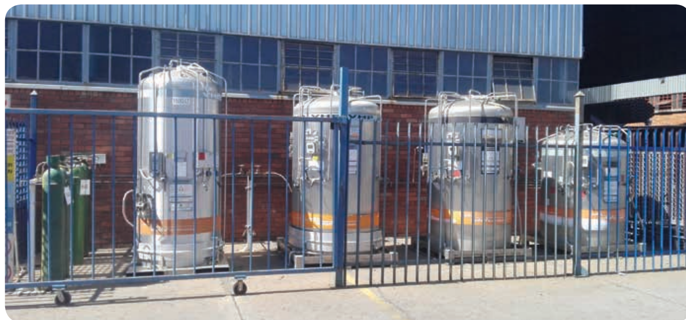
Cost effective, consistent and uninterrupted high volume gas supply is key to making sure that cutting systems achieve maximum up-time and productivity. "At Air Products we focus on this key requirement with special high volume/high pressure installations and innovative high pressure cryogenic liquid delivery systems," says Young.
