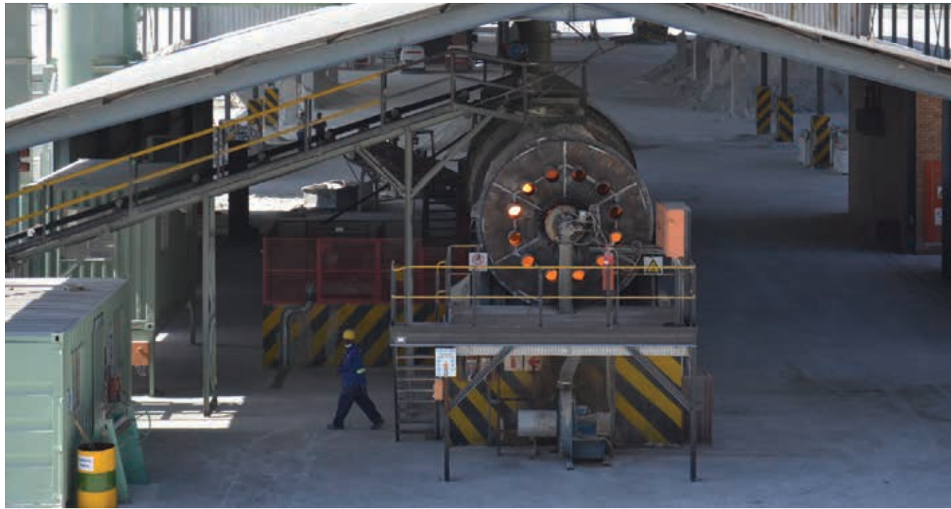
An additional gypsum drying kiln reduces the moisture content of OMV's 20% (post air drying) dihydrate to 10% free moisture.
