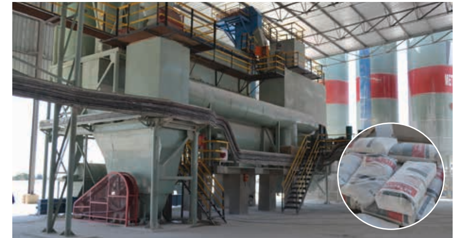
OMV's new Fluidised bed Calcining plant for the manufacture of finished products such as its Metadynamics MetaCote finishing plaster (Inset).
