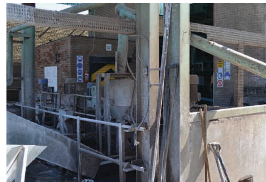
Above: The new automated dosing system takes a pH measurement of a small amount of gypsum entering the system. A computer-based formula is then used to determine the exact amount of lime needed to neutralise this slurry.
