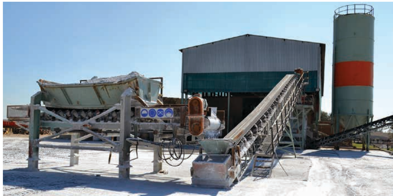
The starting point of reprocessing chemical gypsum is reclaiming the gypsum from the dump and conveying it into the neutralising and washing plant.
