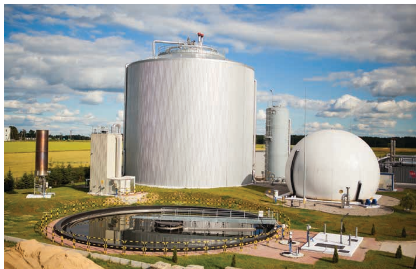
Veolia's Biobulk Completely Stirred Tank Reactor (CSTR) is used by Distell to treat effluent and harvest biogas for use as a fuel.
