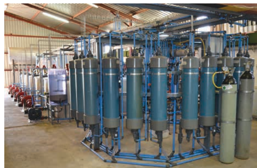
For treatment using the KNeW process, a twin line of stirred tank reactors (CSTRs) operate continuously, with the effluent water flowing from tank to tank. In the foreground is a ring of PLC controlled vessels for regenerating the resins: dilute nitric acid to regenerate the cation resin; and methanol for the anion resin.
