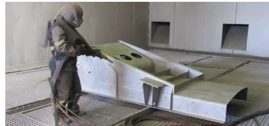
The shot blasting process ready to commence in Kwatani's purpose-built booth. Even the paint specifications come with certificates.
