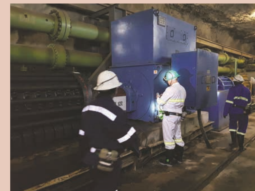
Marthinusen & Coutts technical personnel monitoring the condition of a 3 300 kW pump motor in Zambia at one of the wettest mines in Africa.
