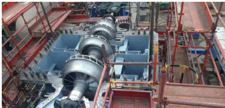
Air Products recently completed a major shutdown at the Sasol Facility in Sasolburg and is extremely proud of the on-time, zero-incident and 100% successful execution.
