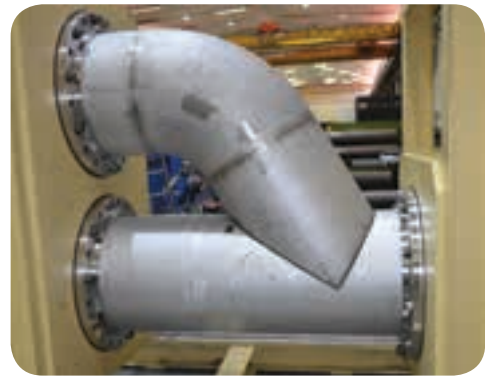
Following careful design of the SEC piping, welding jigs were manufactured for each individual section.
