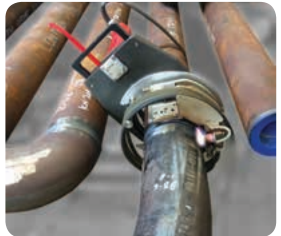
Orbital TIG (GTAW) welding for mild steel pipes being completed using an open type MU Polysoude welding head.
