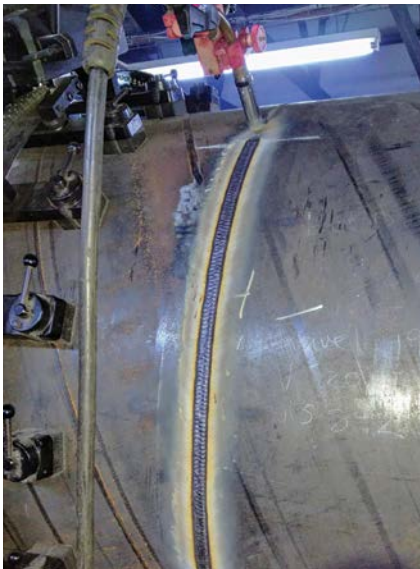
An application trial being done at Renttech's Alrode premises. The root weld is being done using the Böhler Ecospark 420 (ER70S-6) solid wire and the Wiseroot function on a Kemppi welding machine. The fill and cap was then done using the Bohler Diamondspark 46RC (E71T-1M) flux-cored wire using a Promotech Rail Titan welding and cutting tractor.
