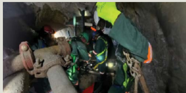
The GammaTech crew is preparing the Elios 3 before launch. The Elios 3 Drone enables inspections in confined spaces to be done safely without putting underground personnel at risk.
