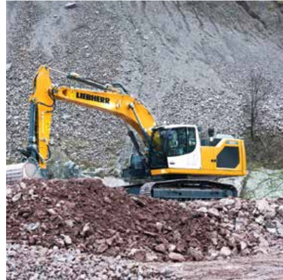
During the lockdown, Liebherr's normal safety procedures for field service and workshop activities are in place in order to achieve zero-harm operations.
