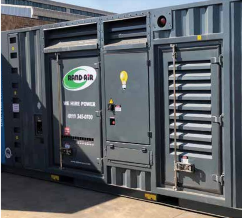
The TwinPower containerised generator from Rand-Air.
