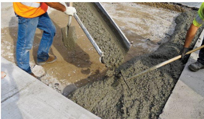
Set accelerating admixtures reduce the time for a concrete mix to change from hardened to plastic state.
