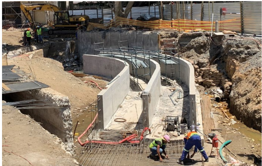
New stormwater culvert with cantilever lateral support in the background supporting the protected tree.
