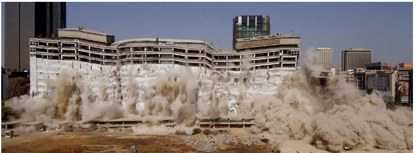
Munitorial building implosion 2013 – another iconic landmark safely and expertly demolished by Draco Group – shaping the future while respecting history.
