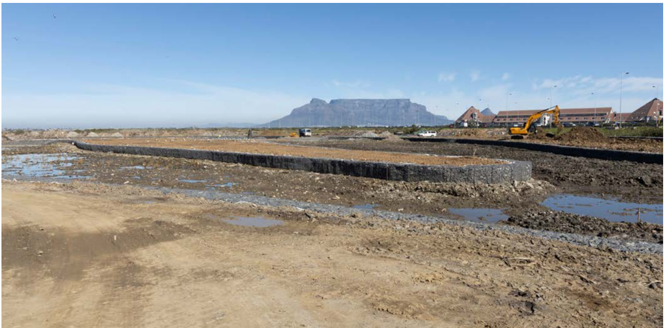
Earthworks have prepared the way for 12 000 m 3 of dump rock for stabilisation.
