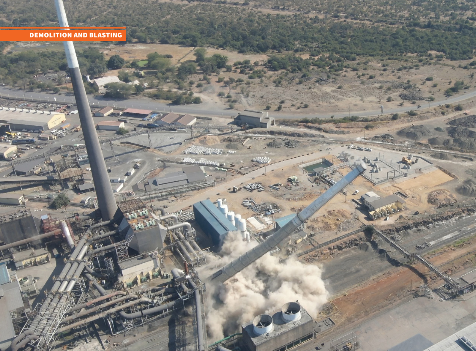
Palabora Mining Company (PMC) - controlled blasting and toppling of 107 m compromised concrete converter stack.
