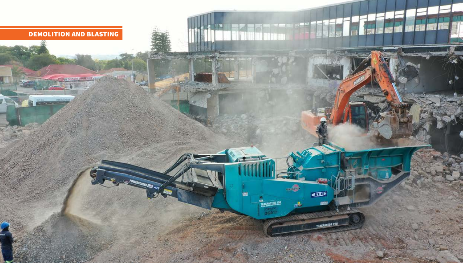
Earthworks in progress at Highlands North – all demolition rubble was crushed to G5 specification and repurposed as backfill, supporting waste reduction and sustainable site rehabilitation.
