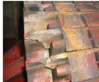
Image 10: Fractured rotor bars.
