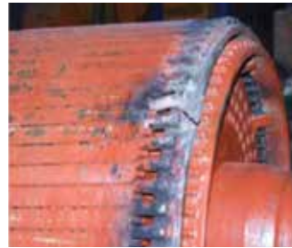
Image 8: Overheating of connections.
