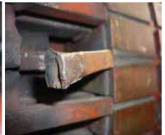
Image 9: Fractured rotor bar showing lamination damage.
