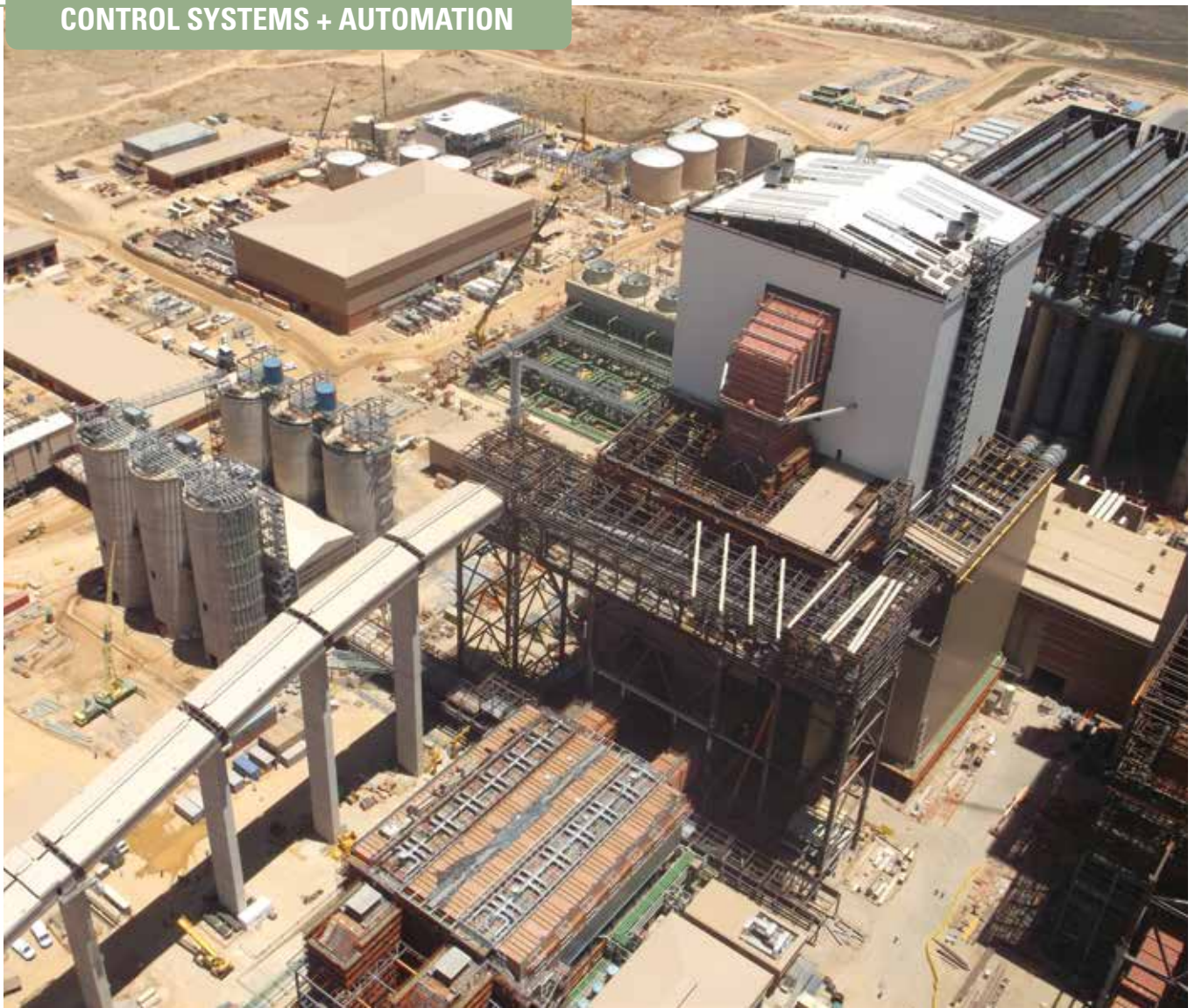
A view of the nearly completed Unit 1 boiler at Kusile, the site of ABB's flagship control and instrumentation (C&I) project.
