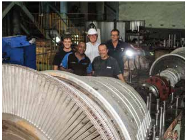
With 57 years of extensive experience, Marthinusen & Coutts was ideally positioned to undertake the turbine refurbishment work at Van Eck power station.
