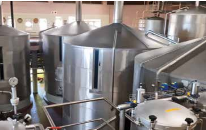
Stainless steel vats in the production plant at Namibia Breweries Limited.
