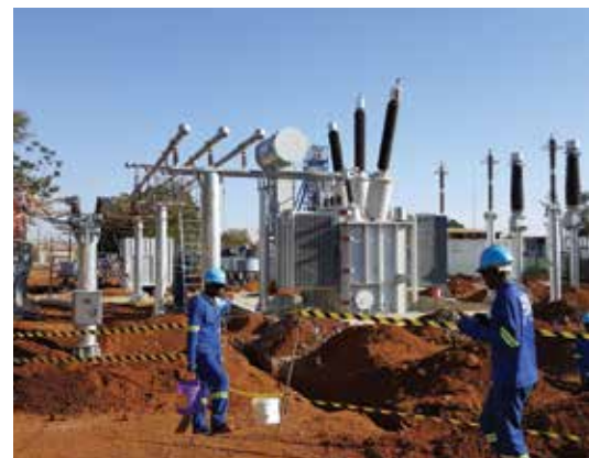
220 kV static VAR compensator.
