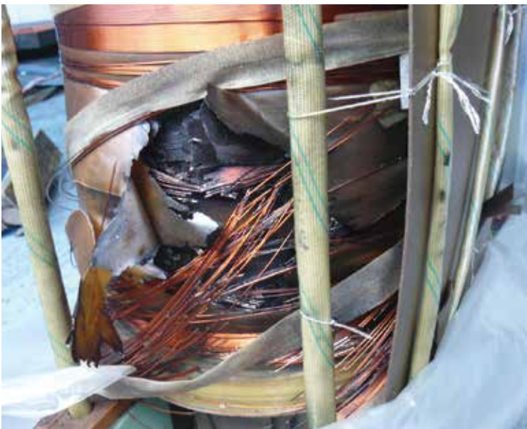
A failed transformer can have a disastrous impact on the operations which depend on it. A good transformer condition monitoring programme detects potential failure before it occurs.
