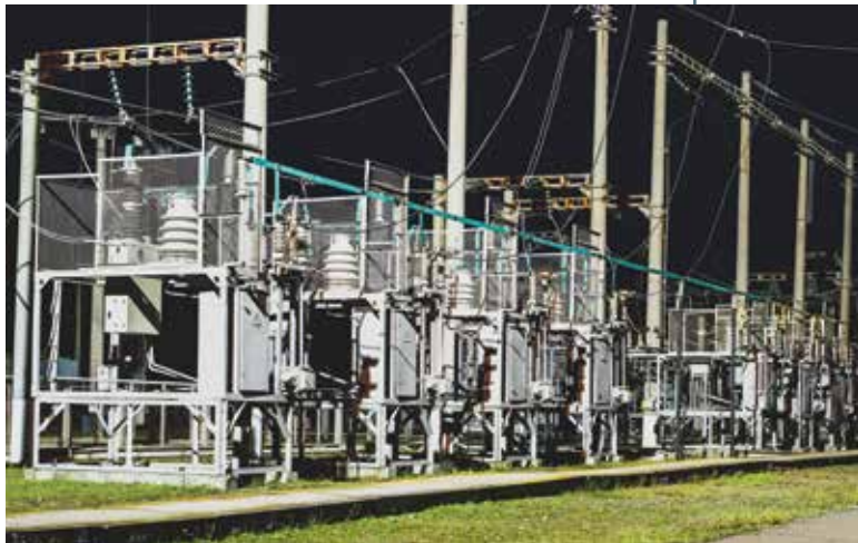
A lack of maintenance on municipal substations and ongoing load shedding from the national grid, raise the risk of substation fires damaging ageing electrical infrastructure.
