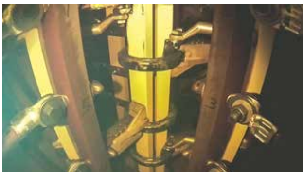
A TXplore high-definition camera view through the transformer's dark oil.
