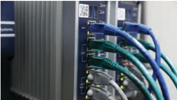
The PROFINET industrial Ethernet protocol enables designers to create reliable industrial automation I/O networks.
