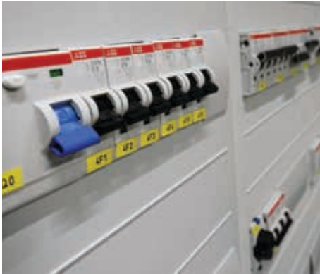
Monitoring the operation of circuit breakers at the substations had been a long-standing problem with no indication if one went off and had reset.
