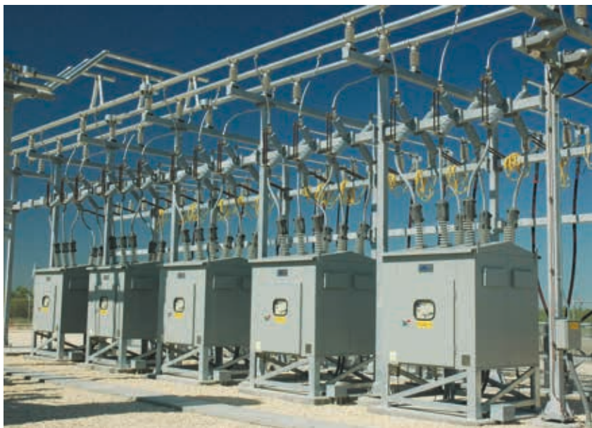
Across the 17 substations on the Natref site, automatically operated circuit breakers are used to protect electrical circuits.
