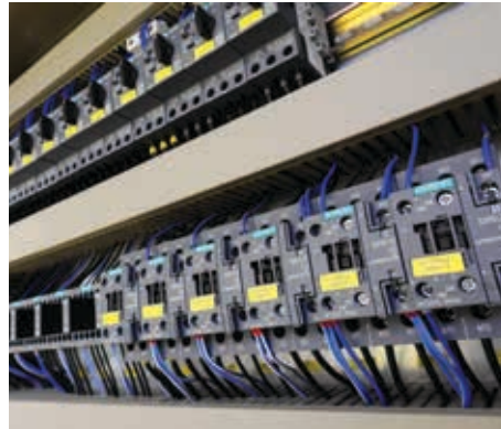
The newly implemented alarm and events logging technology means maintenance engineers can see when an incident has occurred.
