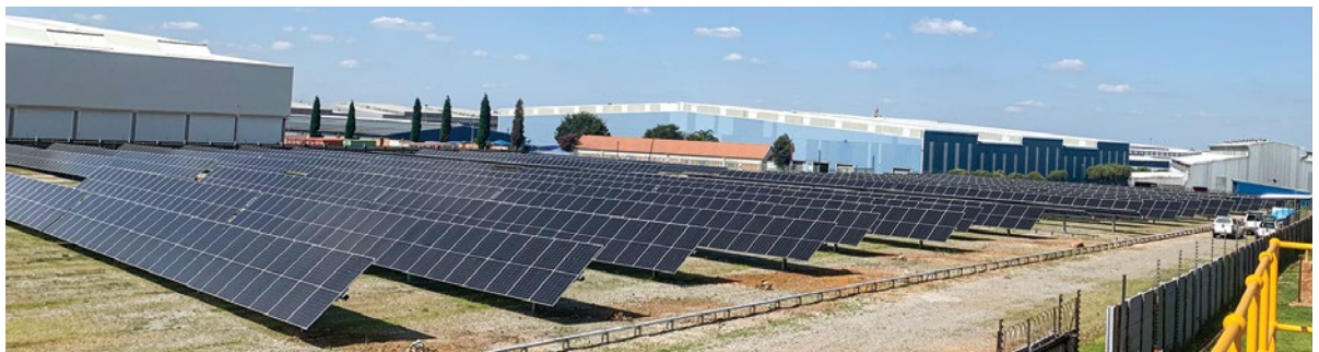
CBI-electric: low-voltage has installed a 1.1 MW solar PV plant at its head office in Gauteng.
