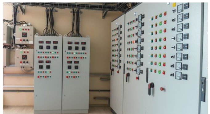
Electrical power management systems provide valuable insights into internal electrical infrastructure.
