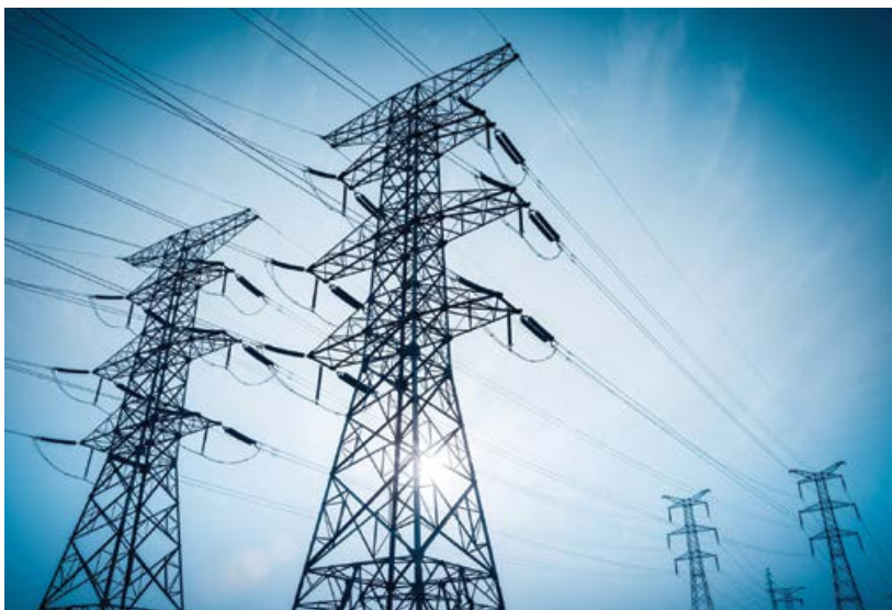
Eskom's updated TDP sees an additional 53 GW of new generation capacity needed by 2032, plus 14 200 km of extra HV transmission lines and 170 transformers.
