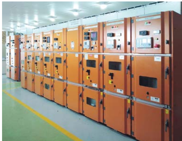
ABB's Unigear switchgear line-up at the Syferfontein substation.
