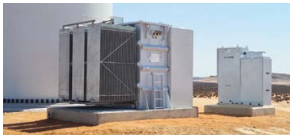
One of the padmount 2.7 MVA 0.69/33 kV inverter transformers produced for the wind turbines of the Kangnas wind farm in the Northern Cape.
