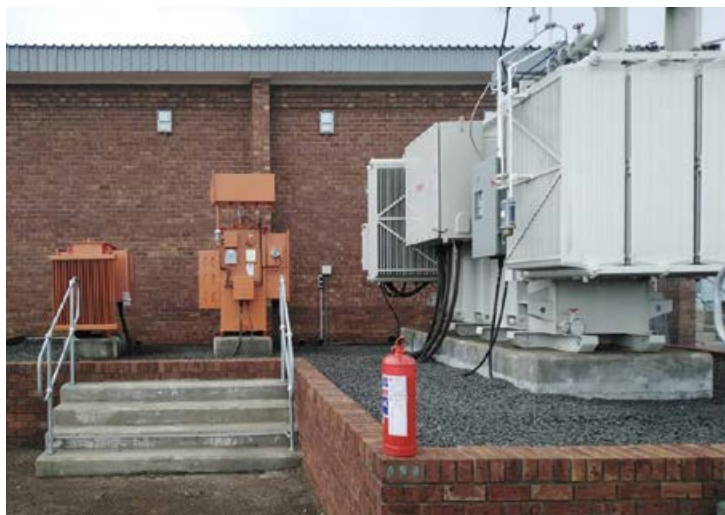
An external view of the substation.
