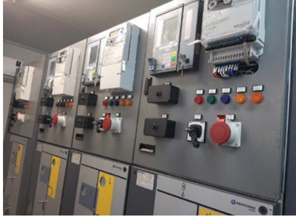
By design, safe and quick MV switching is possible at any site.
