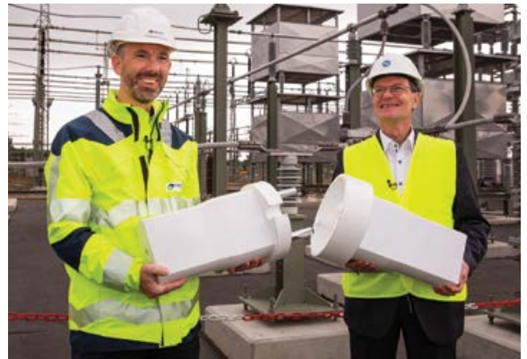
TenneT Germany and MR recently symbolically commissioned the new MSCDN plant.
