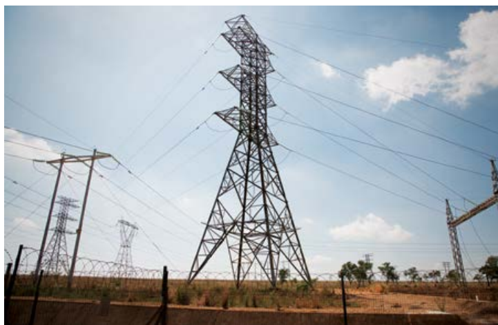
Recognising constraints on transmission networks in some parts of the country, Eskom plans to accelerate investments in developing new corridors and substations.
