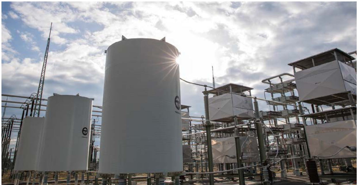
The Schwandorf substation is a key regional supply node.
