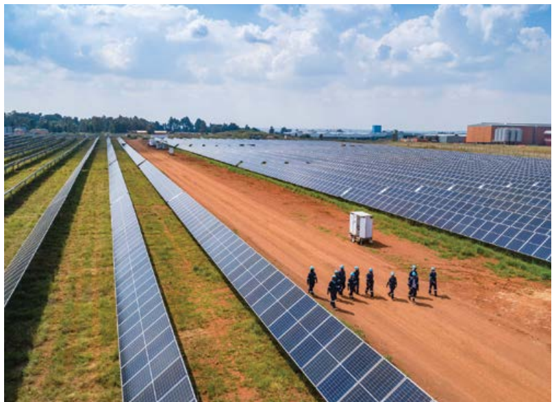
With 14 000 panels and covering a land area of 19 ha, the solar plant has an energy capacity of over 6.5 MW.
