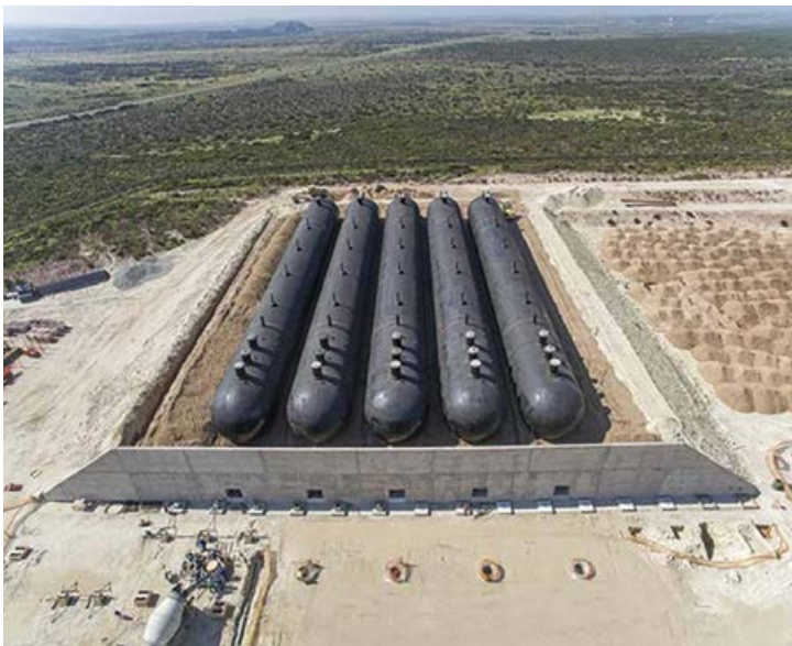
At Sunrise Energy, some 5 500 metric tonnes of explosive LPG are stored in underground 'bullets' that are protected using impressed current cathodic protection (ICCP).
