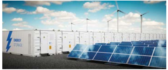
Combined with renewable energy generation, battery energy storage provides the stability of supply required to meet baseload demand.
