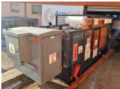
The skid substations are transported on low-bed trailers to the mining sites where they can be quickly energised.
