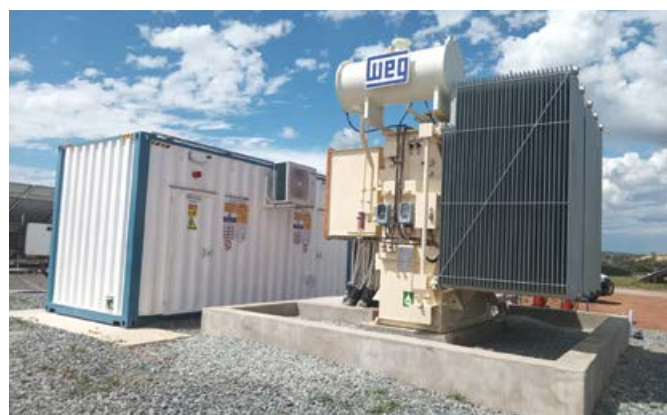
The WEG photovoltaic solution: the company supplied 10 x 5 MVA, 11 000/600-600 V transformers with ester oil as the coolant.
