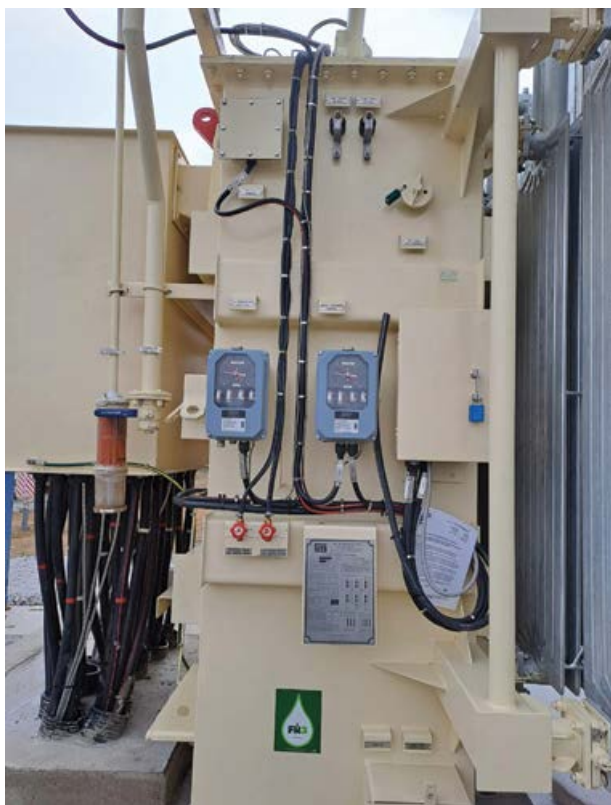
A view into the PV transformer shows some of its key components.
