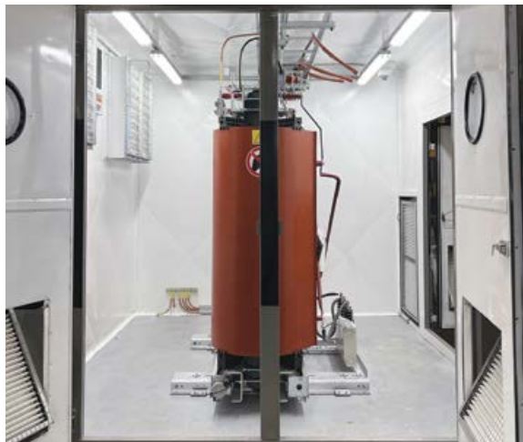
The use of dry-type transformers in a modular substation offers additional advantages.
