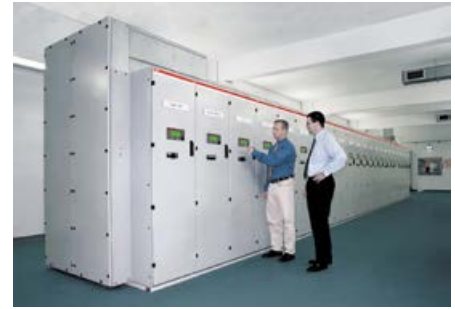
ABB's 33 kV GIS switchgear is now 60% locally assembled, to global standards, by Eya Bantu.
