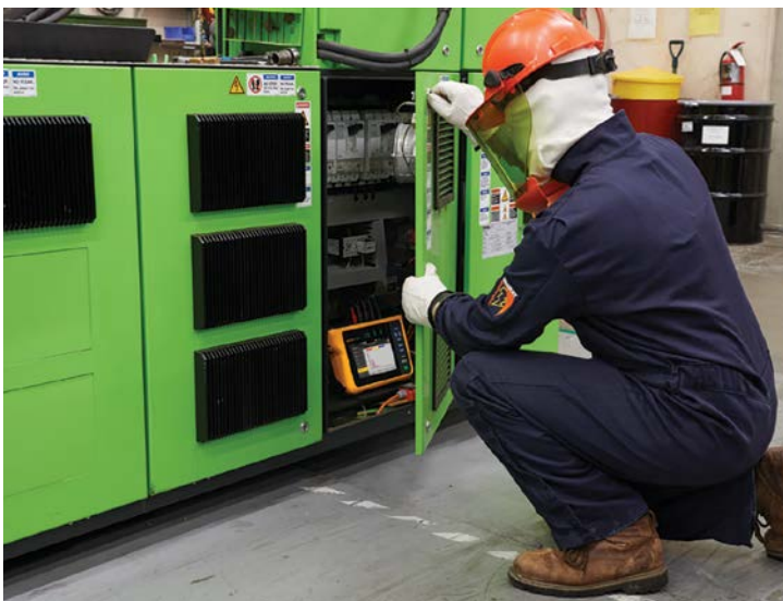
Using power quality analysers, energy managers can locate energy waste and act to gain energy savings.
