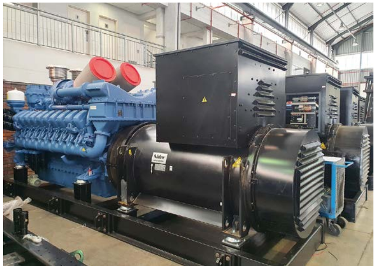
3 000 kVA 400 V primary equipment before being installed in its enclosure.
