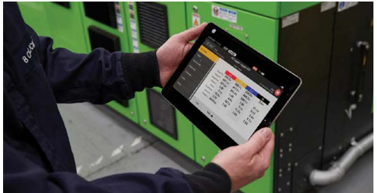
Monitoring power consumption with the Fluke 1777 three-phase power quality analyser.
