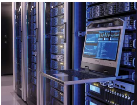
As demand grows for edge data centres in offices, factories and warehouses, suitable cooling is essential for each installation.
