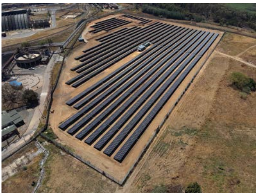
AECI has successfully commissioned the 4 MW solar park adjacent to its Modderfontein facility.
