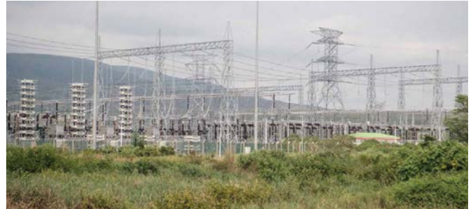
The HVDC electricity interconnection between Ethiopia and Kenya represents a technological advance for electricity transmission in the region.
