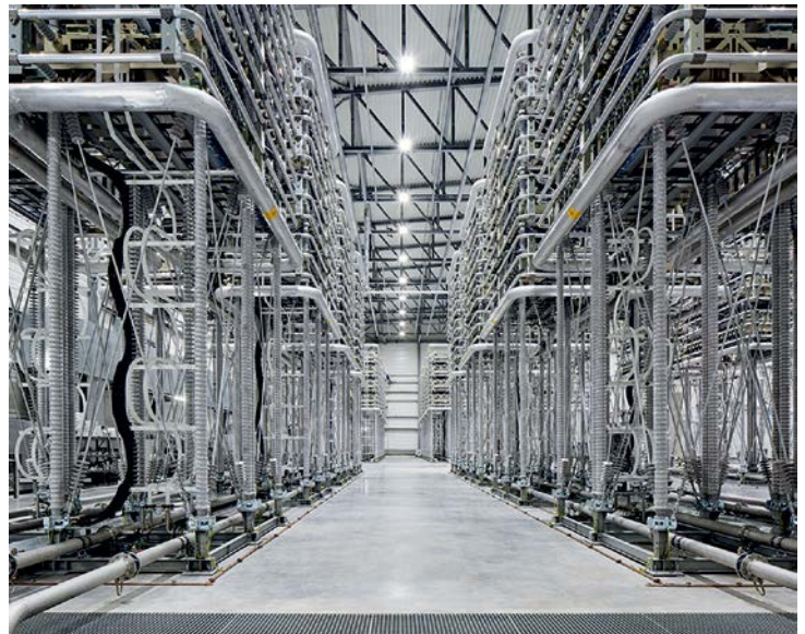
As a manufacturer of systems for energy transmission and stabilisation of the power grid, Siemens Energy puts its trust in PC-based control technology from Beckhoff (in this case: a system for high-voltage direct current transmission).
