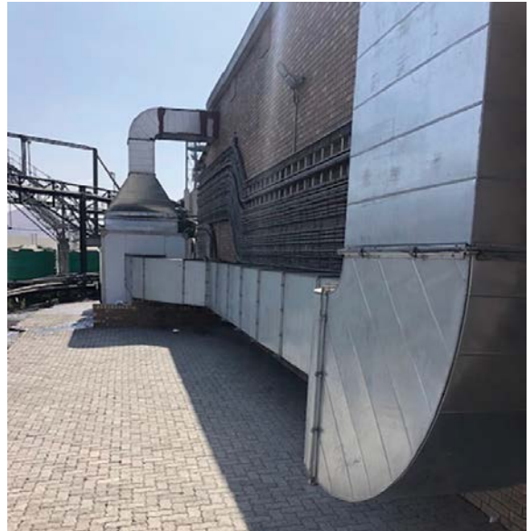
Iritron is working with leading HVAC suppliers to offer customers a full suite of IoT integration options for HVAC systems.
