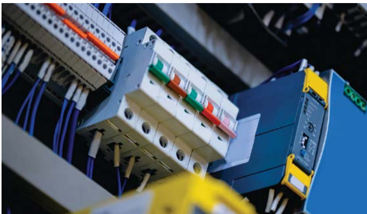
Using a pre-configured electrical panel can have a positive impact on productivity in the setup process.
