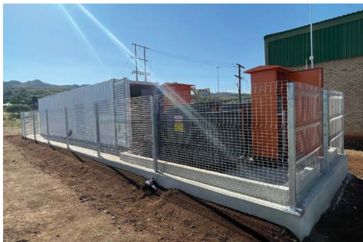
The containerised battery energy storage system at the Clapham Pumping Station in Limpopo.
