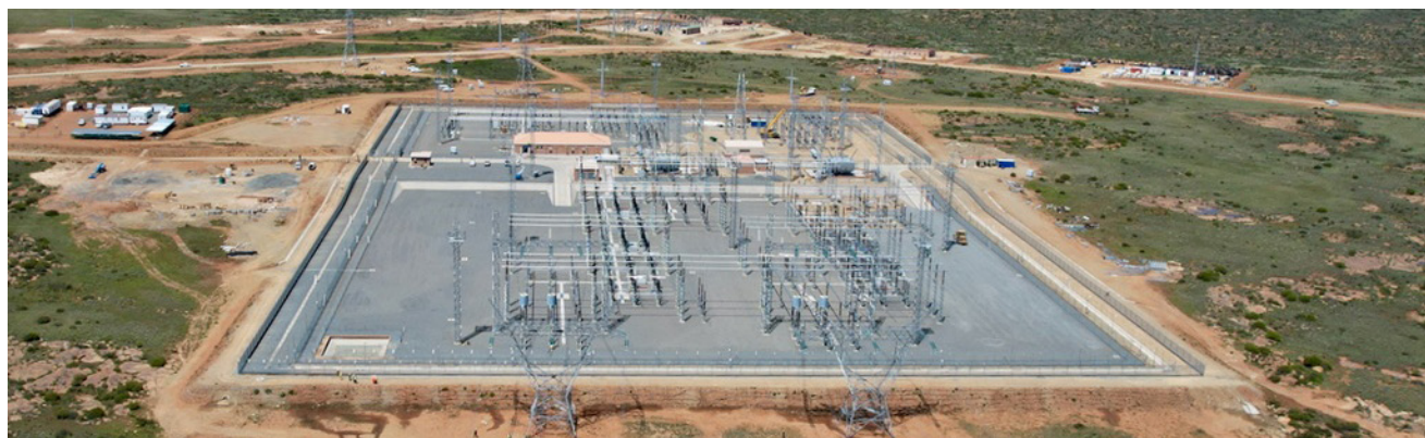
EDF Renewables has commissioned the Koruson main transmission substation.
