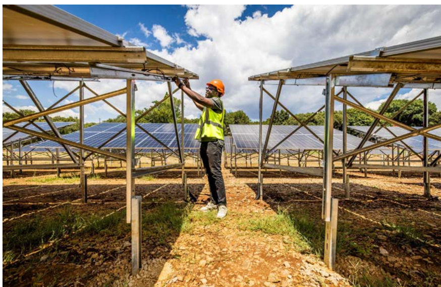
Candi Solar offers assessment, optimisation and ongoing maintenance to ensure solar installations perform as specified.
