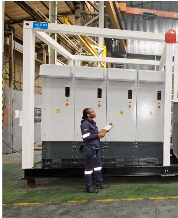
An Integrated MV Transformer and Inverter Station in production at ACTOM Power Transformers.
