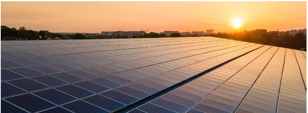
Among the critical factors that influence power generation capacity and cost effectiveness in utility-scale PV plant centres on how the modules are set up on the site and the use of fixed tilt or single-axis tracking modules.
