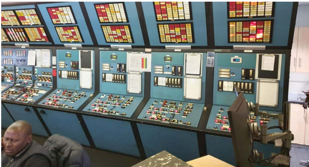
Omniflex today provides a central monitoring solution that covers three Sasol sites.
