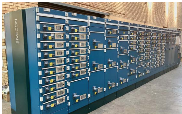
A Hamar Controls 3 200 A Siemens SIVACON S8 MCC supplied to an industrial client in South Africa.
