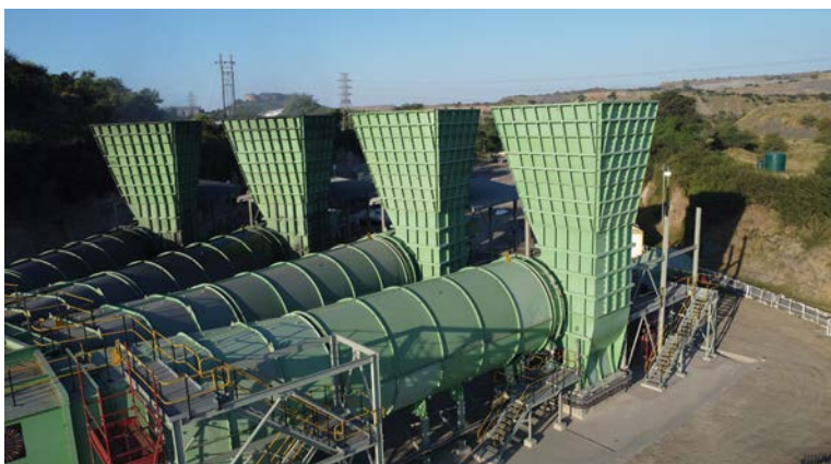
The ventilation fans installed at the mine each stand about 15 metres tall and 7.2 metres wide.
