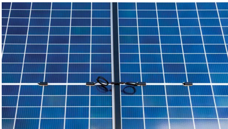
While it continues to provide training on solar PV installations, PQRS also offers a range of technical energy management services.
