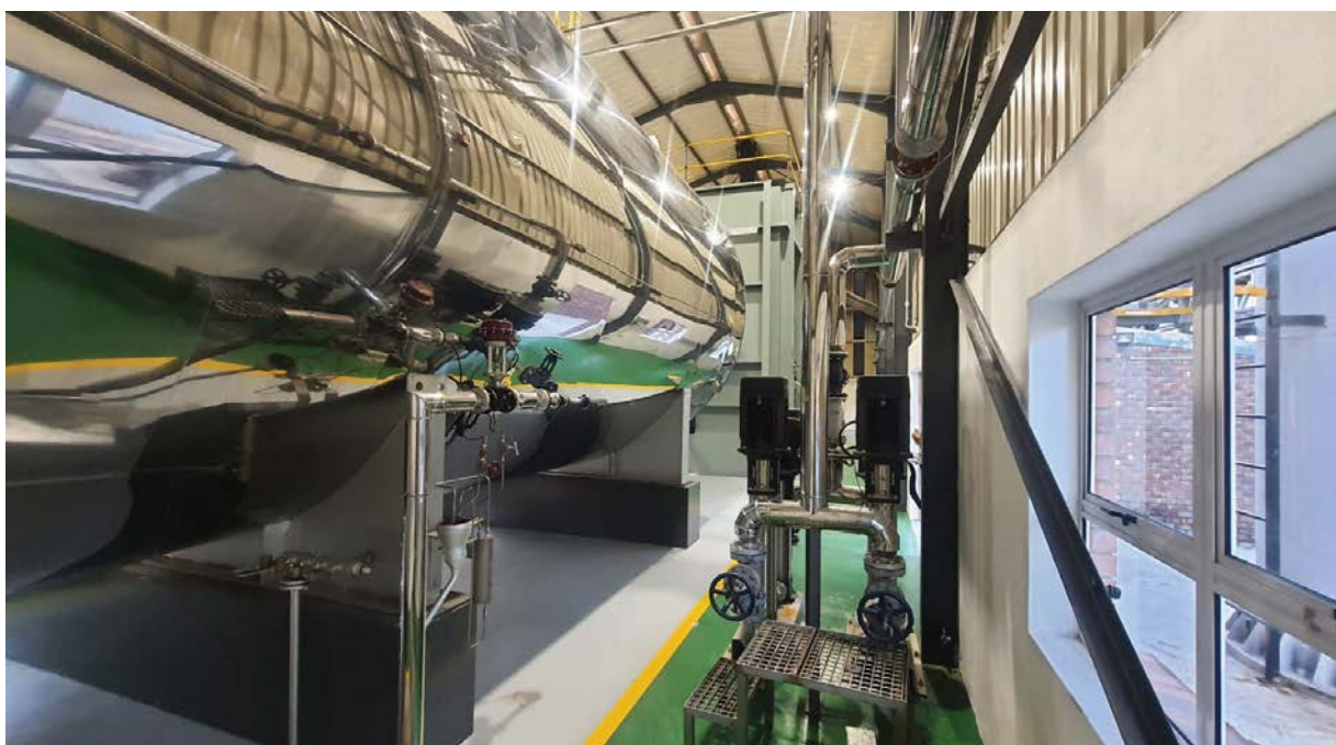
AES biomass boiler at a multi-user site using three fuel types.
