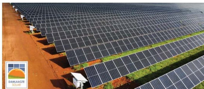
The Damlaagte solar PV facility located near Parys in the Free State is now in commercial operation.
