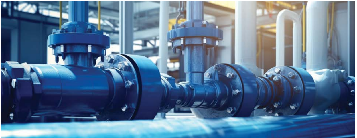
Among other infrastructure sectors, ABB supports water utilities by providing advanced solutions to optimise water distribution networks.
