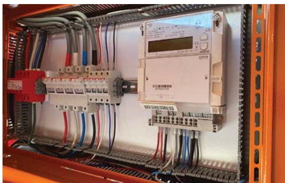
All cabling has been carefully routed to minimise interference and allow for easy maintenance access.
