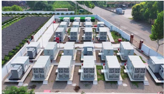
The 150 MW agrivoltaic + storage project powered by Trina Storage’s Elementa Series.
