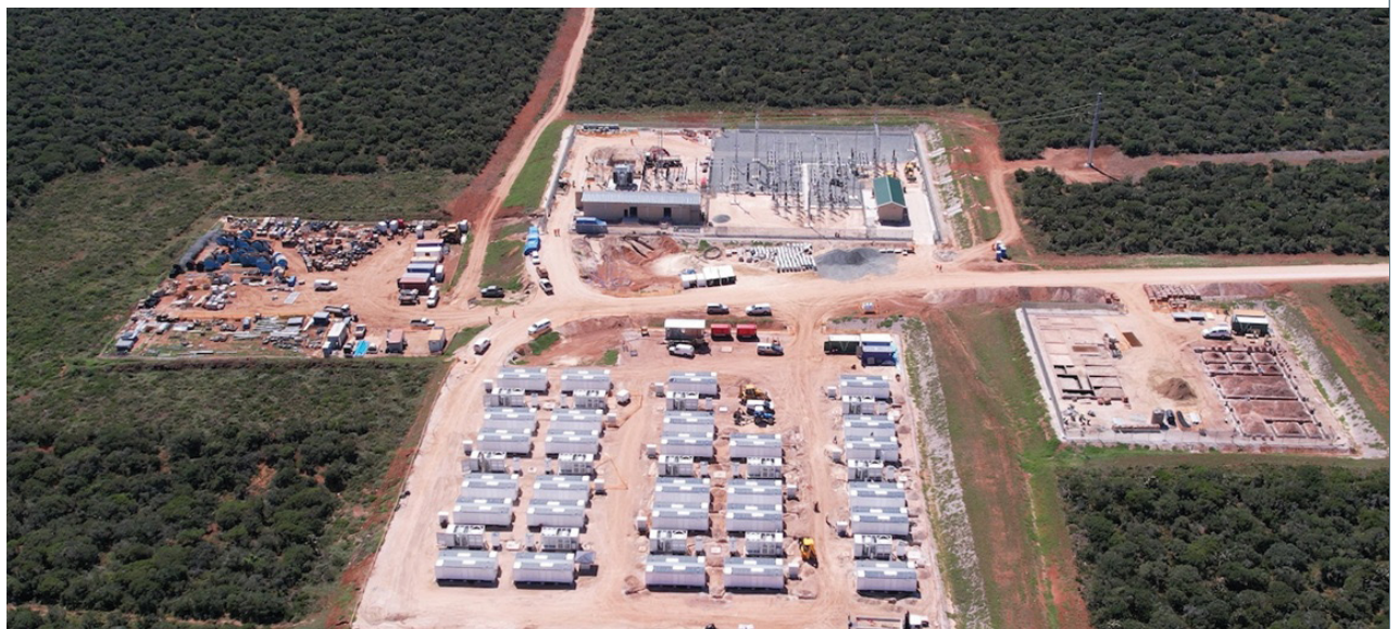
Battery energy storage and the main transmission substation at Umoyilanga Dassiesridge.
