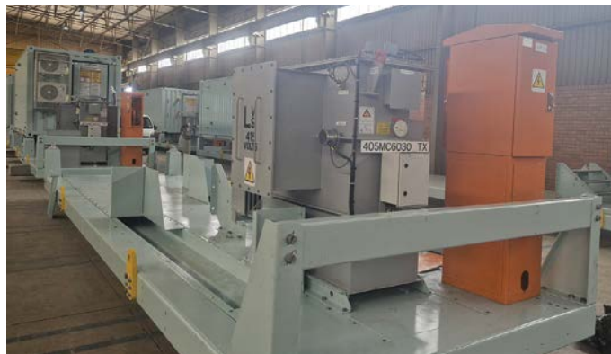
Trafo Power Solutions has provided nine transformers to a mineral sands operation in Mozambique; seven were skid-mounted so they can be easily repositioned on site as needed.
