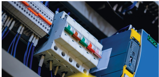
Quality is critical for the safe and efficient performance of electrical cables.
