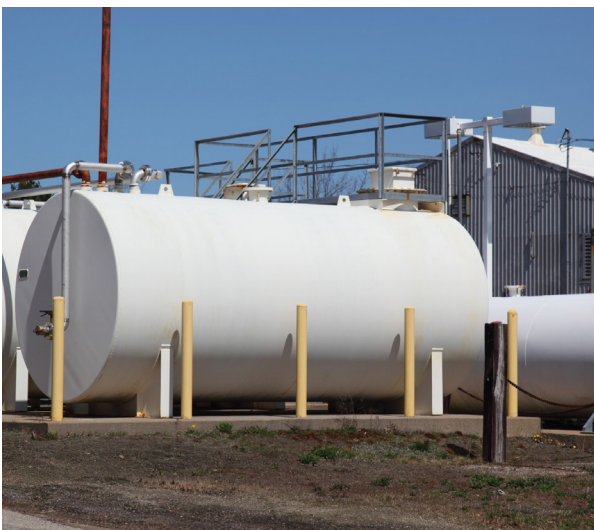
Above-ground petroleum storage tanks present a particularly high fire safety risk and require specialised fire protection systems.
