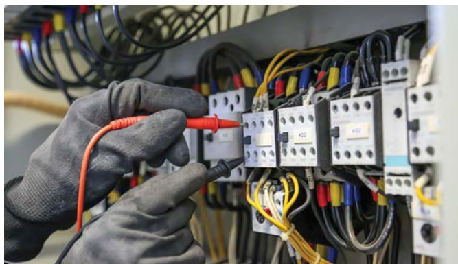
Where legacy power quality meters have not kept up with evolving electrical systems, retrofits can be straightforward.
