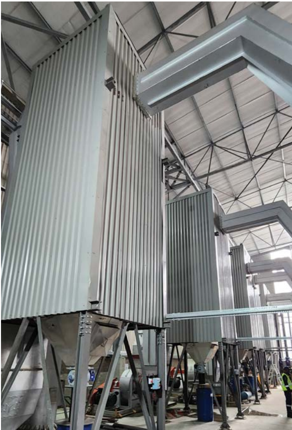
A high efficiency multi-cyclone helps mitigate particulate emissions.
