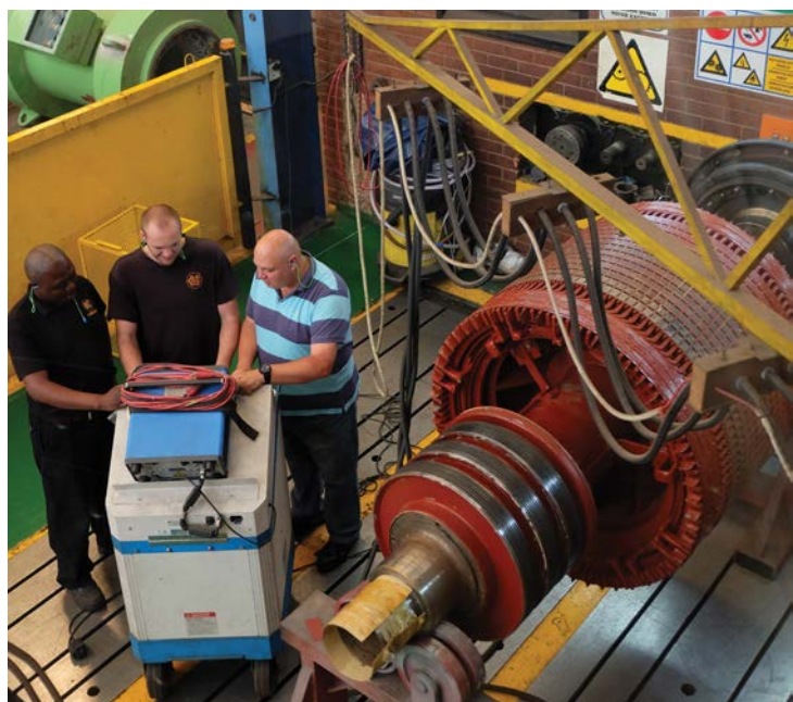
M&C offers full load testing of HV, LV and dc equipment, and on-site diagnostics.
