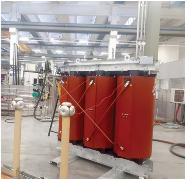
Partial discharge testing is conducted to verify the integrity of the insulation system and confirm the dry-type transformers' compliance with performance and safety standards.
