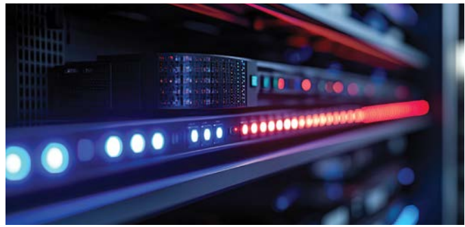
The exponential increase in AI workloads is forcing data centres to increase computing power, in turn raising energy use, heat generation, and the need for more efficient cooling.
