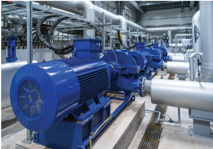
It was clear that the Vyeboom pump station needed an upgrade, but it needed to be completed within a narrow shutdown window to ensure farmers would have reliable water when the season opened.
