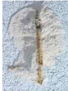
Figure 9: Unprotected aluminium down conductor – incorrect installation.
